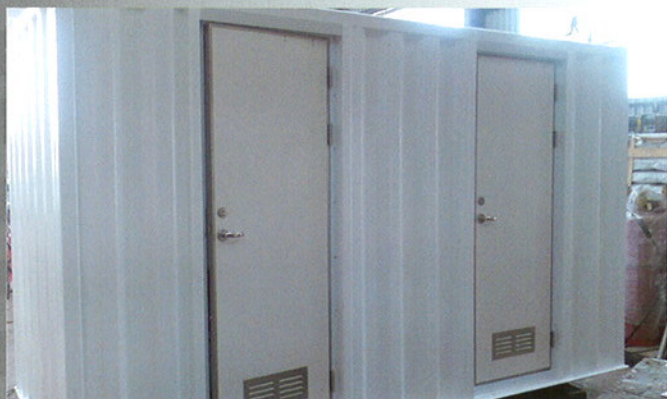
PANNA MUKHTA BATTERY ROOM
